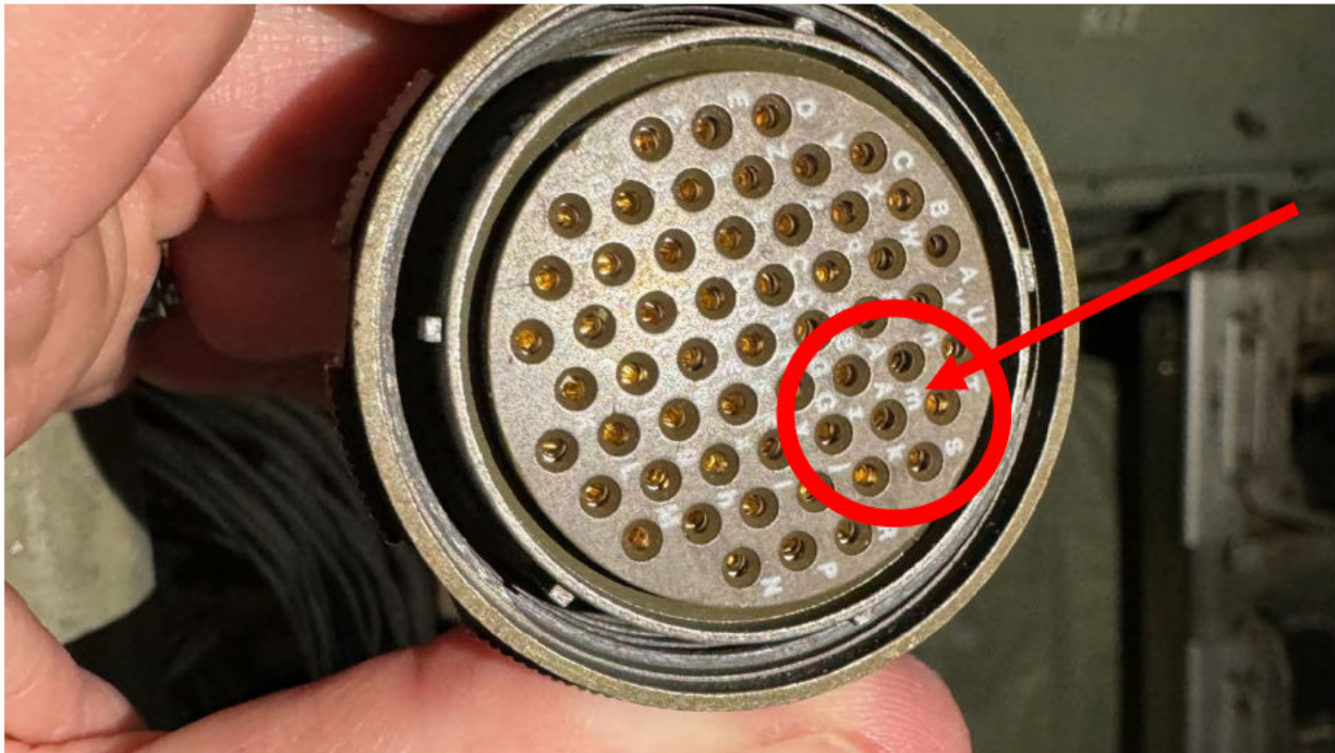
Intermittent fault detected by the PIFD due to a recessed connector receptacle (Pin 36, "little m")
