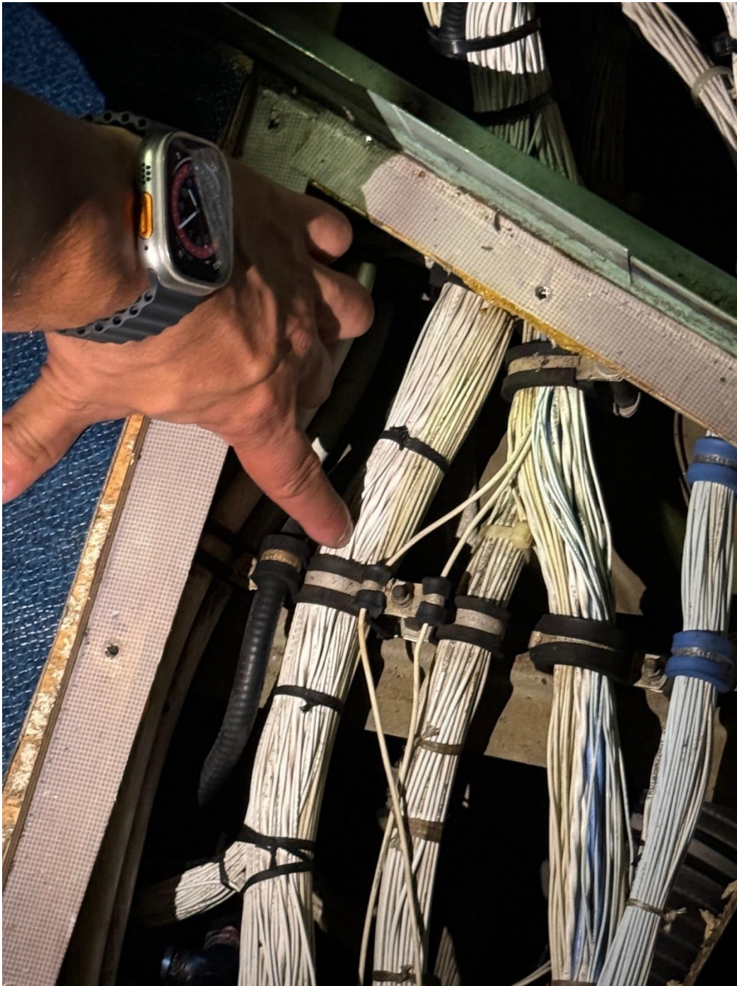
Cockpit location of the wire harness and the location of the detected and isolated intermittent wires. The intermittent wires are located next to the mounting clip.
