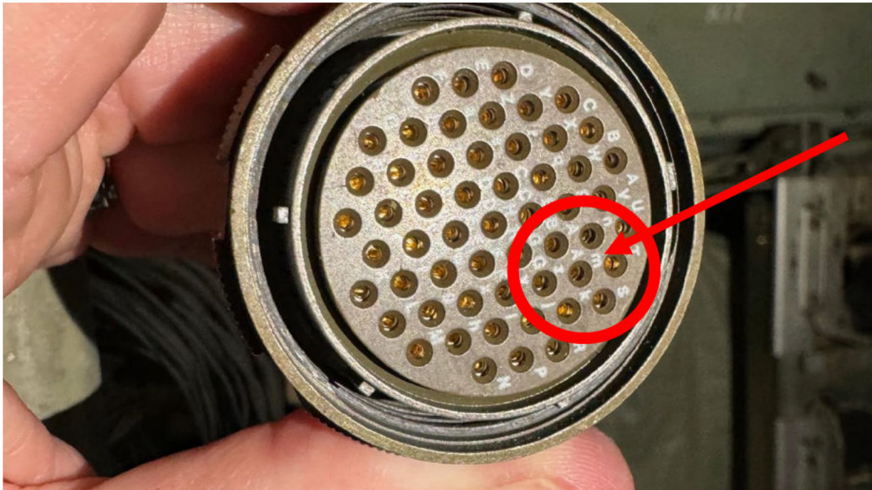
Intermittent fault detected by the PIFD due to a recessed connector receptacle (Pin 36, "little m")
